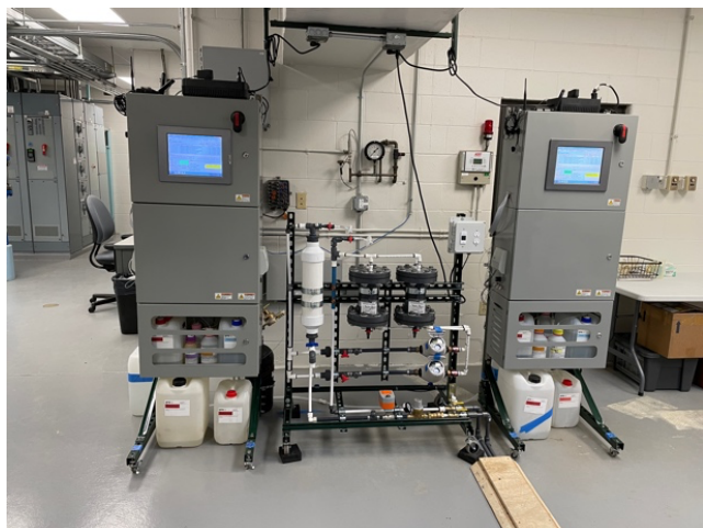
Figure 1- MetalGuard PRS Corrosion and Metals Release Risk Alert System Installation at Madison, WI.
